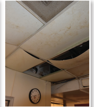
Leaky Roofs and Damaged Ceilings
